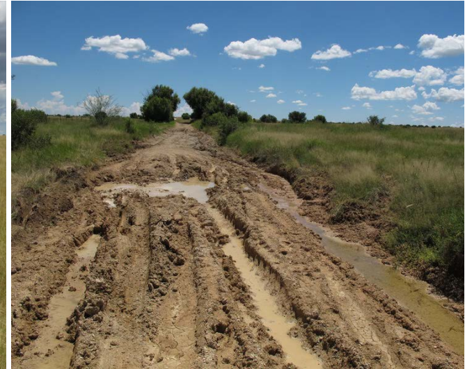
Fig. 9. Access road washed away (A. Sliwa)
